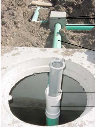
Septic Tank, D-Box and Zabel Filter
