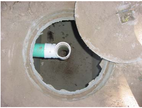
Septic Tank – Outlet (Liquid side)
