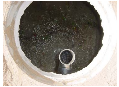
Septic Tank – Inlet (Solid side)
