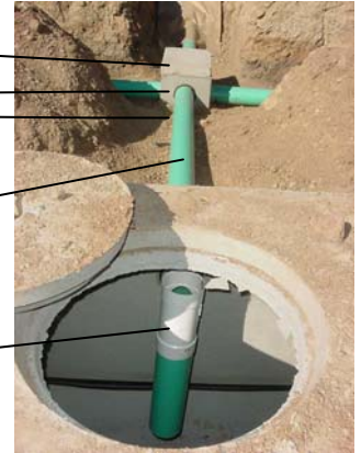
Septic Tank, D-Box and Sanitary T
